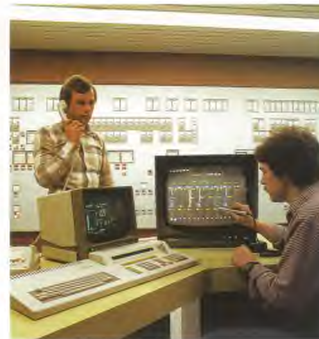
A new process control system handles process operations. Video terminals equipped with light pens
